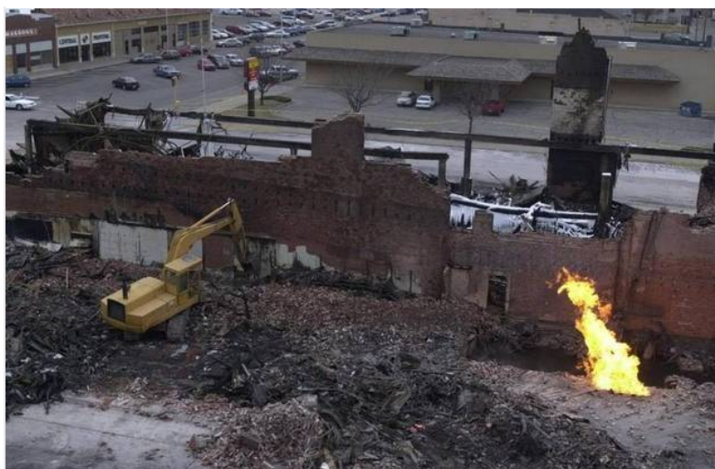
Figure 8. Photo of downtown Hutchinson, KS, after explosion from an underground storage field at Yaggy
